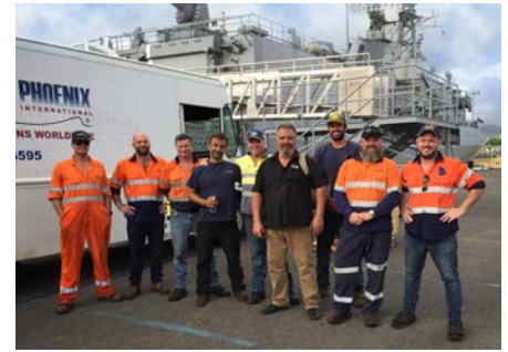
Babcock PM Team with Specialist Support from IKAD and Phoenix during in-water propeller shaft bearing replacement in Hawaii
